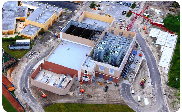
Aerial Photo of the Central Energy Plant (Zone 4), NSU
