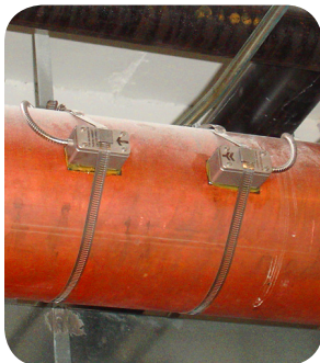
Flow Transducers on Chilled Water Pipe
